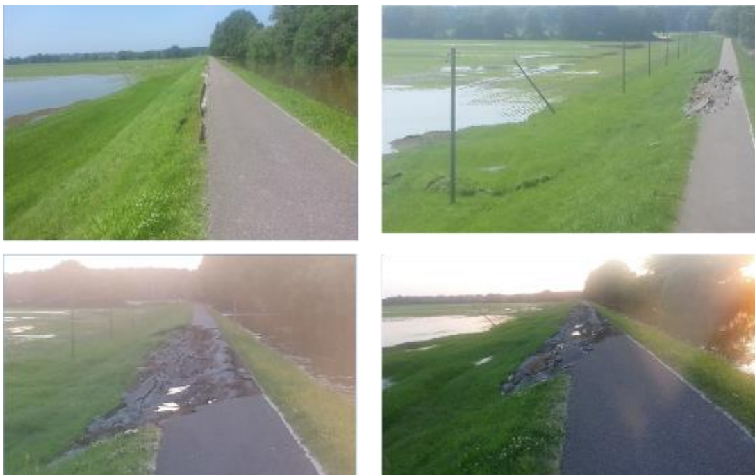
Time-lapse of the Breitenhagen levee failure along the River Saale in Germany, 2013. (from Grubert, 2013; see Kool et al, 2019).
