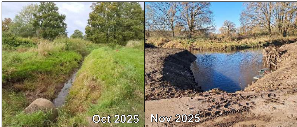
Figure 2: Images of tributary mouth before and after tributary mouth widening intervention in field site 1. The site is located on the River Dinkel in the eastern Netherlands. Construction occurred in October 2025. Both photos taken from approximately the same position.
