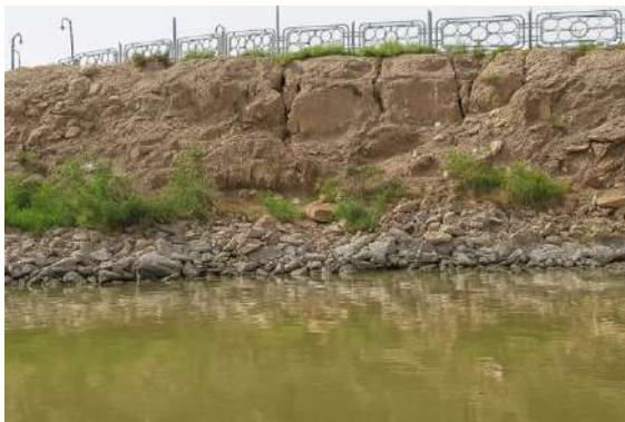
Figure 2. The collapse of the protection measure in Al-Nuaamaniyah location.
